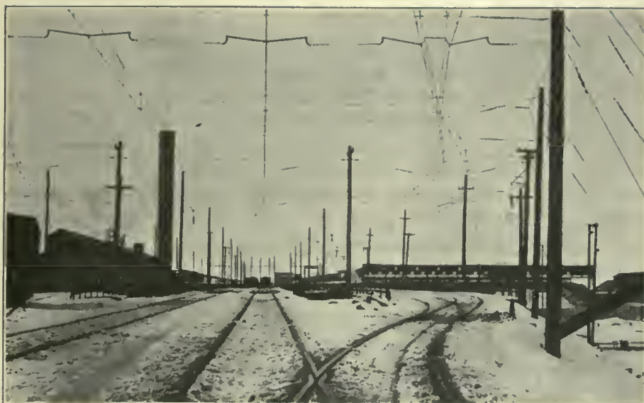
FIG. 529. OVERHEAD CONTACT SYSTEMS. Single Catenary 2,400-Volt Direct Current Yard Track Construction, Butte, Anaconda & Pacific Railway.
